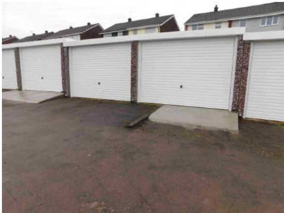
Covered gutters get blocked surfaces
