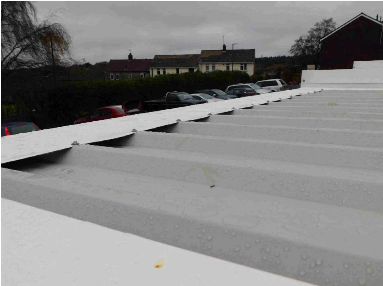
A competitors gutter systems, hard to clearout see garage on Page 16
