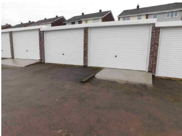
Covered gutters get blocked surfaces
